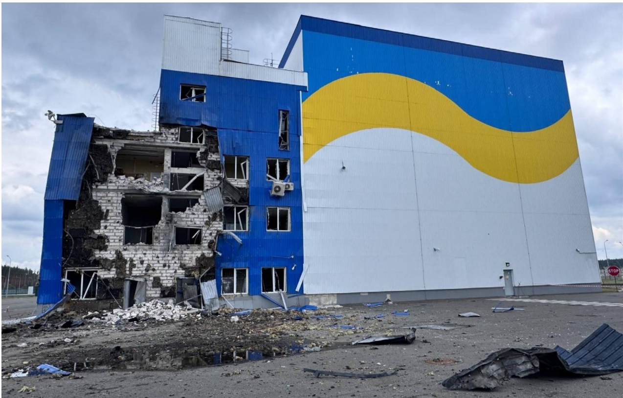
Damaged building of the Centralized Spent Fuel Storage Facility (CSFSF).
