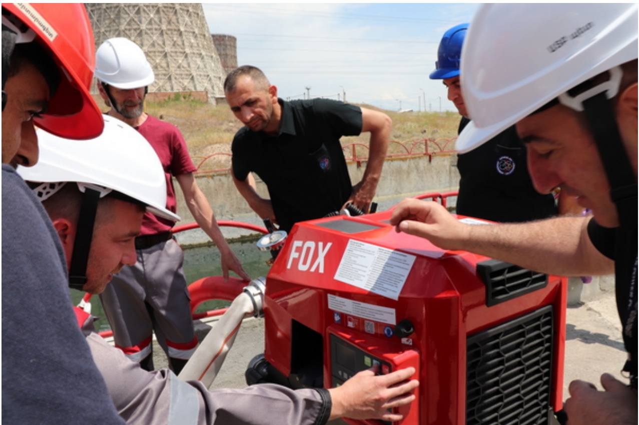
Alternative emergency water supply equipment delivered to the Armenian NPP.
