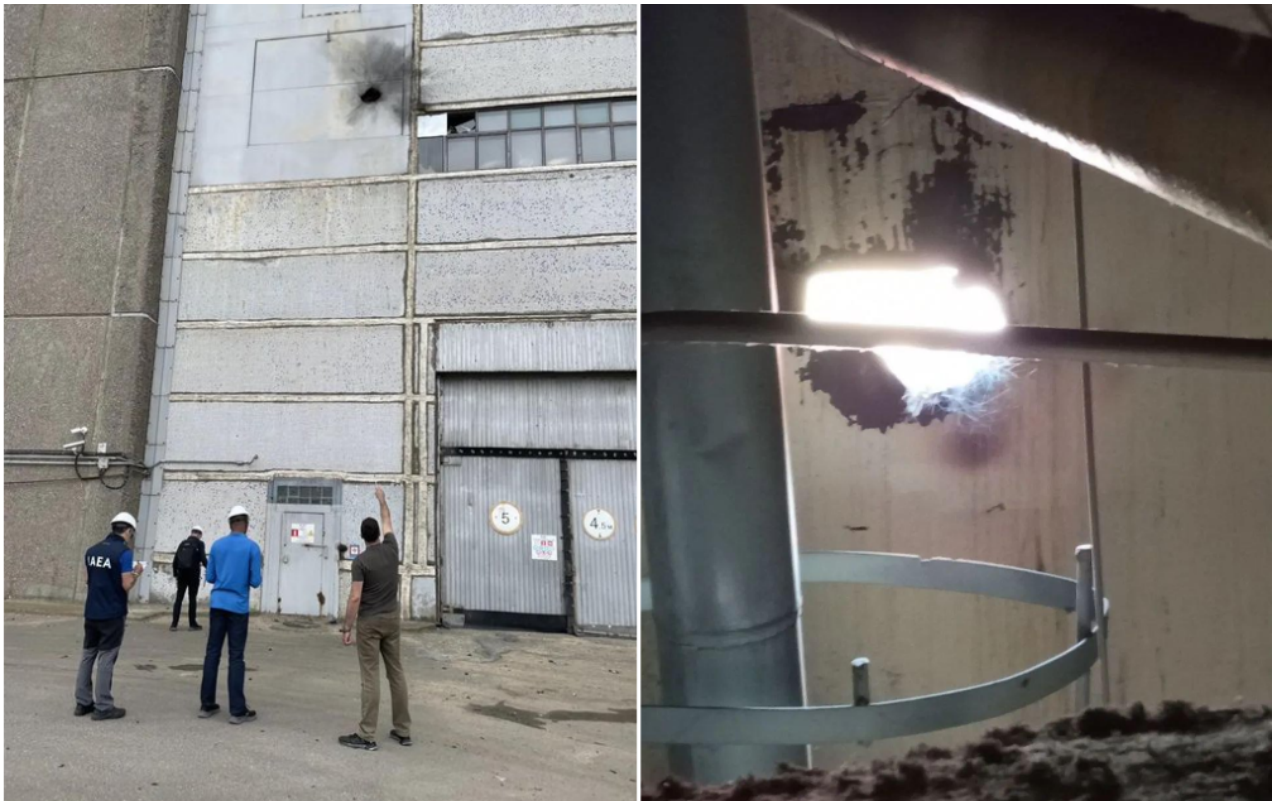
IAEA experts inspect damage to the wall of the Unit 6 turbine hall at the ZNPP. Credit: X / Mikhail Ulyanov (1, 2)
