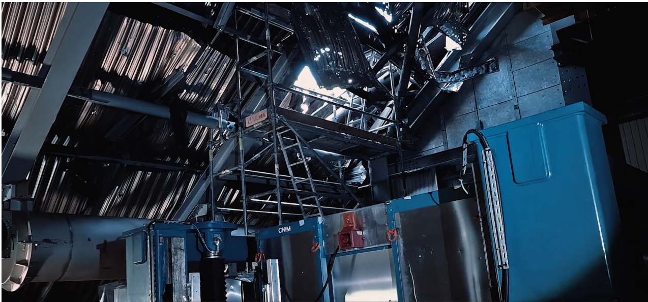
Drone strike impact site on the New Safe Confinement over Unit 4 at Chernobyl NPP. Credit: EBRD video screenshot
