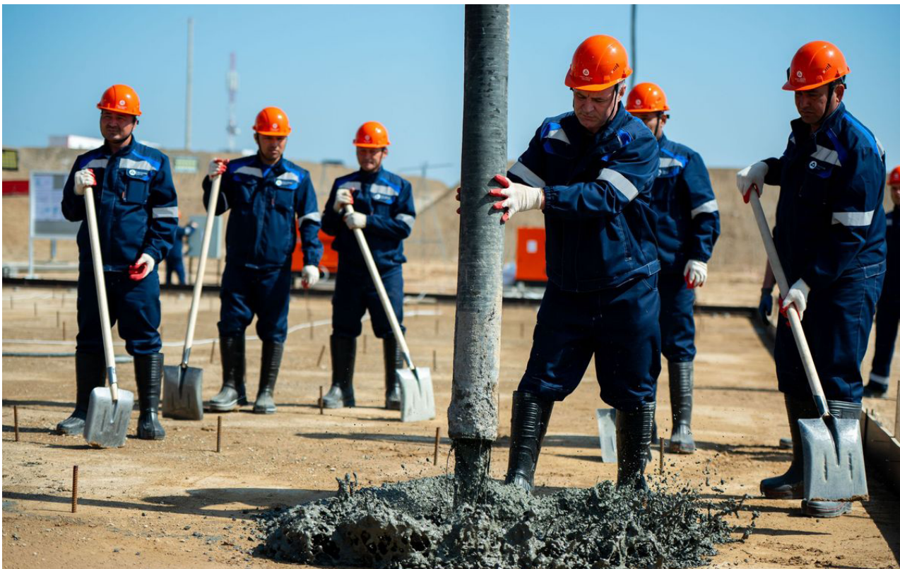
Start of concrete works as part of the construction of a small modular NPP in Uzbekistan.
