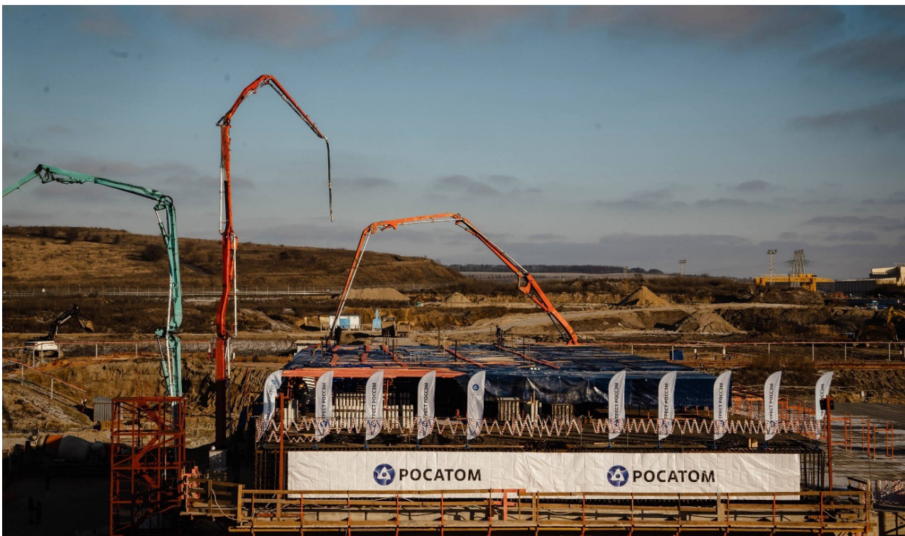
Photo from the first concrete ceremony for Kursk NPP-2 Unit 3, from the Telegram channel of Kursk Region Governor Alexander Khinshtein
