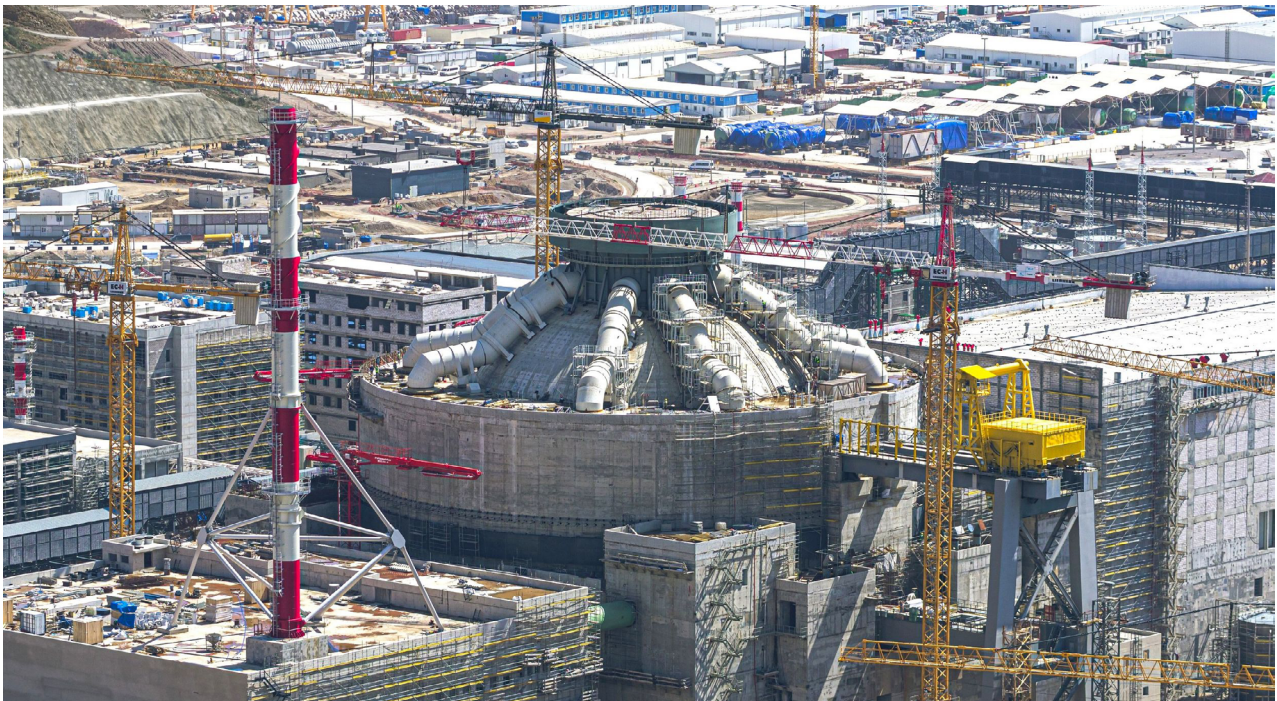
Passive heat removal system at Unit 1 of Akkuyu NPP.
