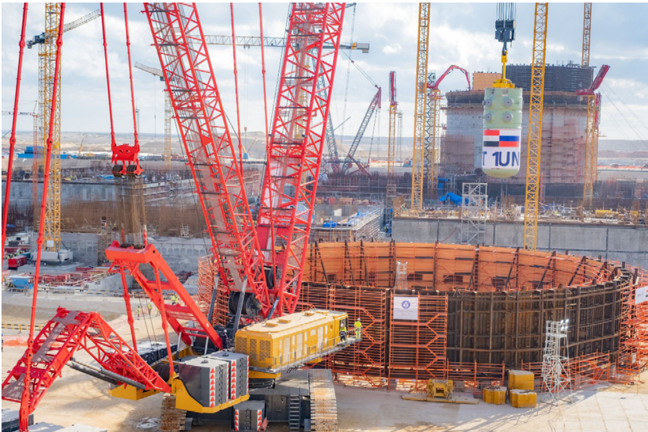
The reactor vessel for Unit 1 is installed in its design position at the El Dabaa NPP construction site in Egypt. Source: Atomstroyexport
