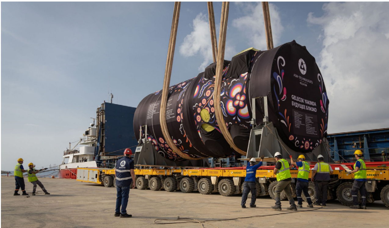
Delivery of the reactor vessel for Unit 4 to the Akkuyu NPP construction site. Source: AtomMedia 183 Sanctions and project delays in 2025
