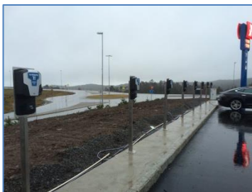
Lillesand charging station with eight charging points
